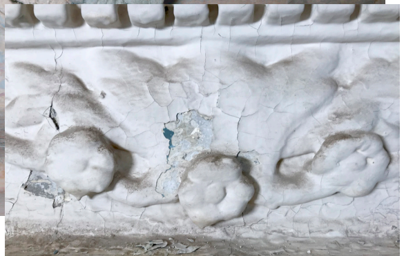
Before treatment conditions
