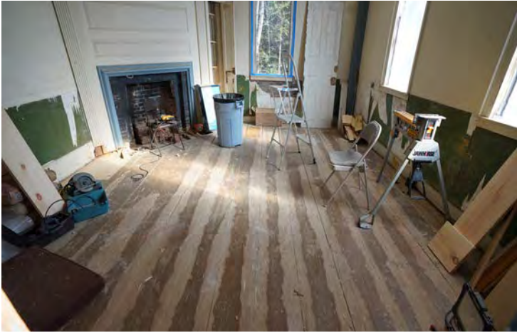
Parlor floor conditions before treatment
