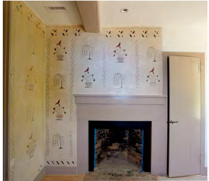
Kitchen Chamber after treatment
