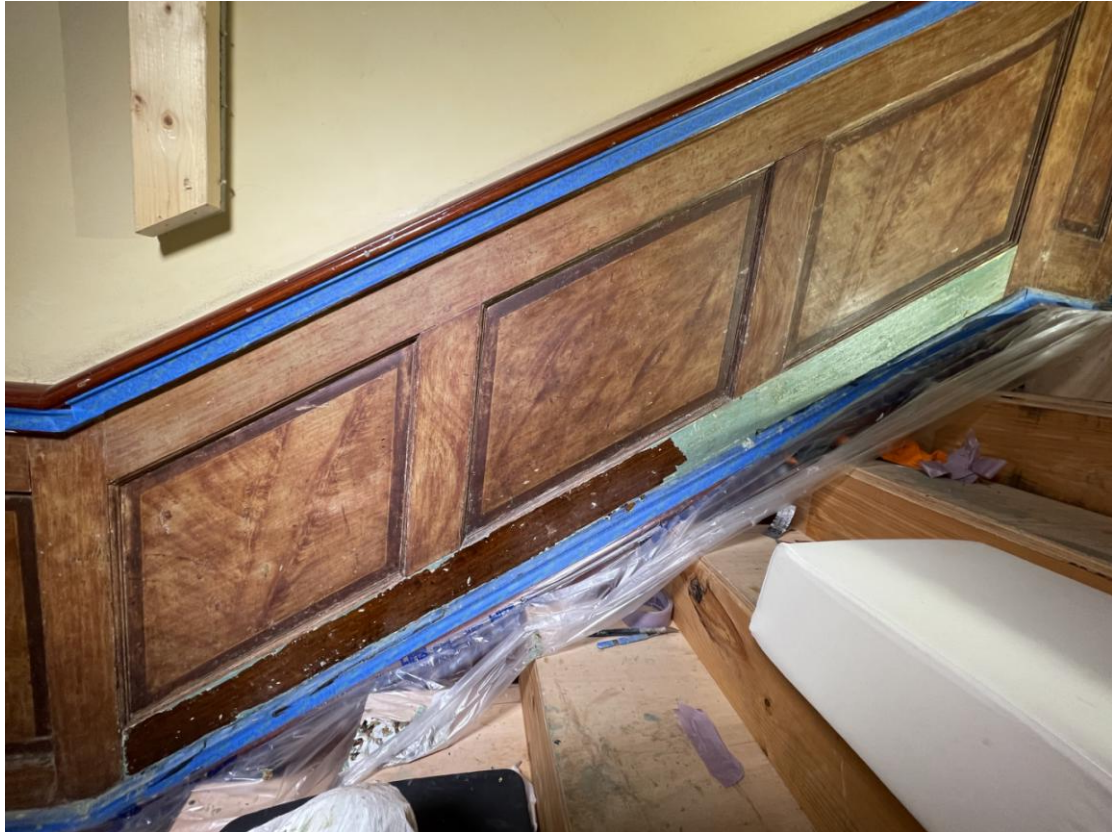
Image 31: The wainscoting that parallels the stairs from the first floor to the landing. The second graining campaign layers are missing in the very light areas (Source: Taylor Day, 2022).
