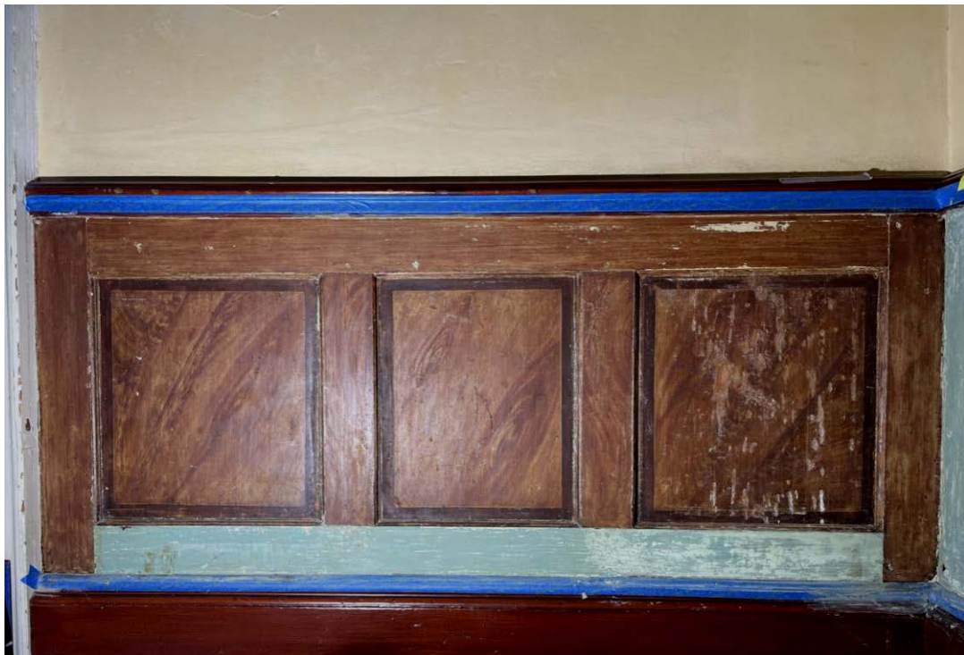
Image 32: Wainscoting on the stair landing. The panel on the right is the most heavily damaged among all of the Stair Hall panels (Source: Taylor Day, 2022).
